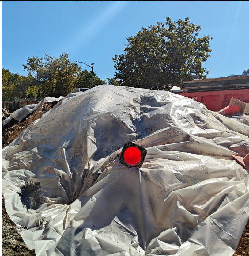
Photo 4- Representative photo of covered stockpile at the end of the day's activities.
