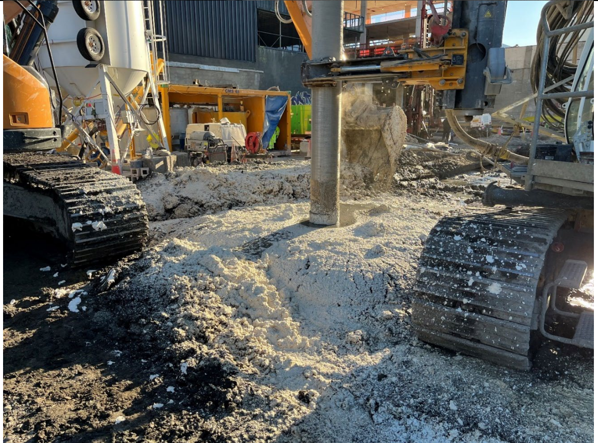
Photo 2- Representative photo of ATMOS Application on Column 186.
