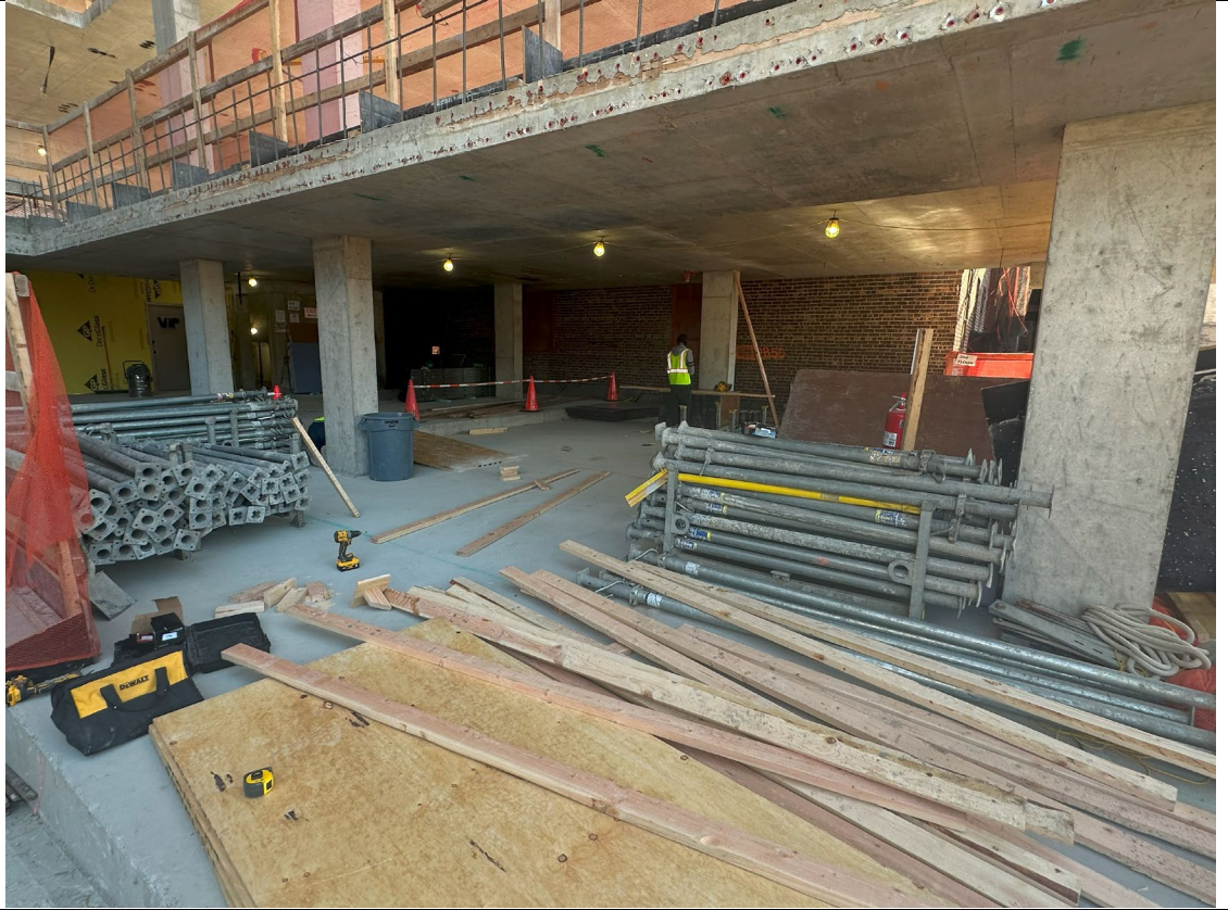
Photo 4- Representative photo of second floor work for portion of building along Butler corridor.
