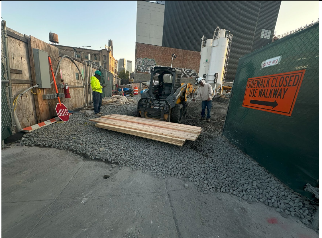
Photo 2- Representative photo of equipment tires being washed before exiting Site over track pad.
