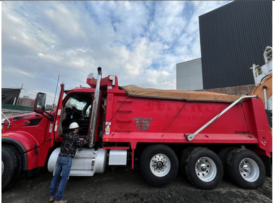
Photo 2- Representative photo of swell truck cover securely strapped down prior to departing the Site.
