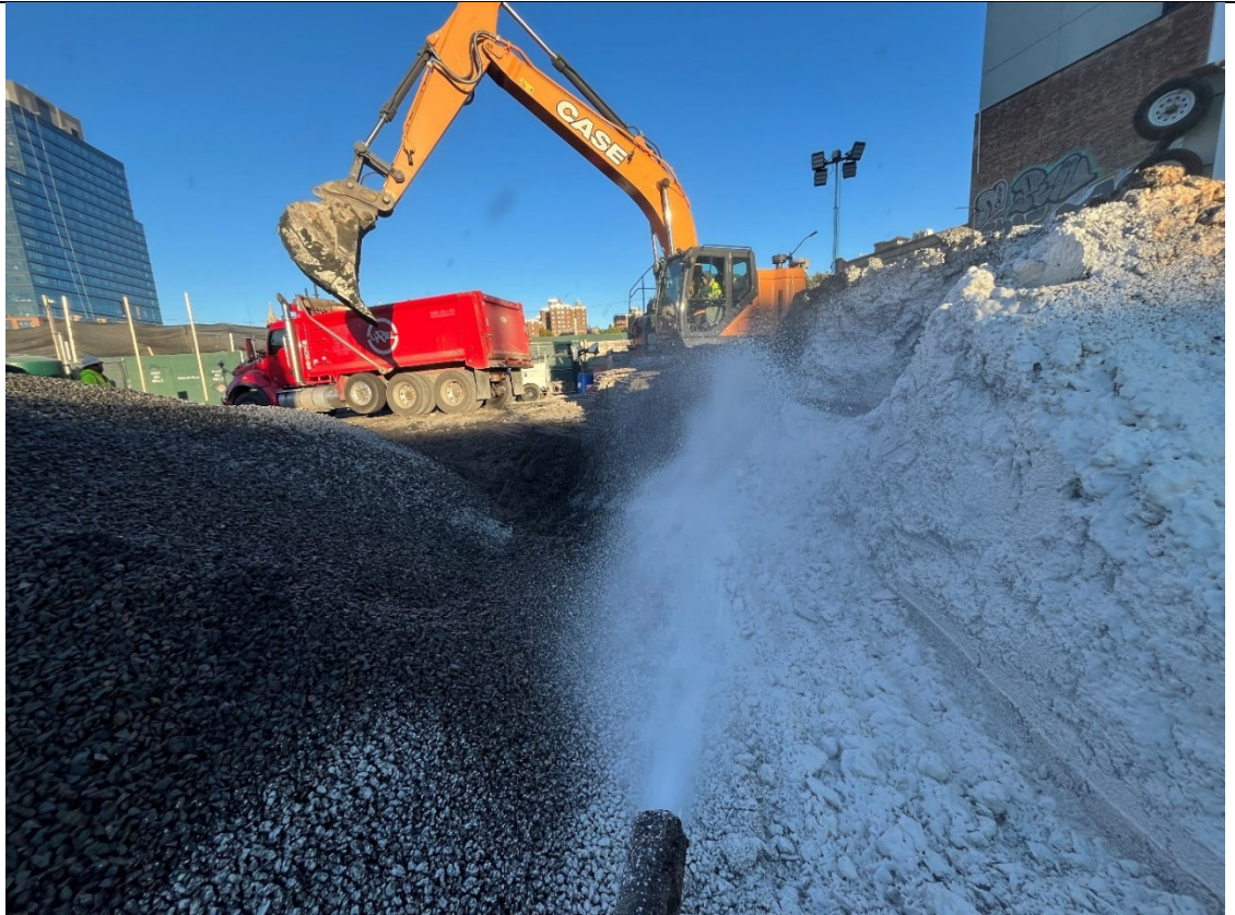
Photo 1- Representative photo of ATMOS application to swell material during loadout of material.
