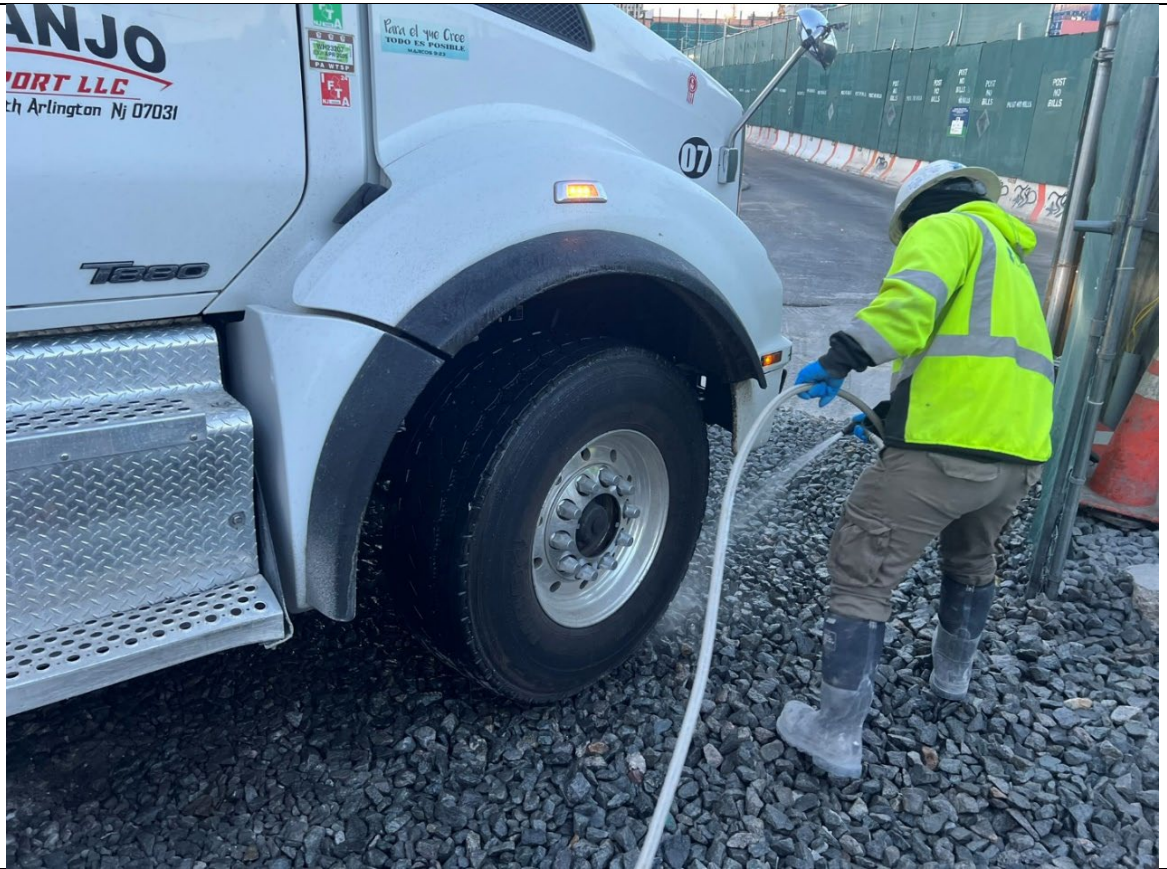
Photo 3- Representative photo of washing tires over track pad prior to exiting the Site.
