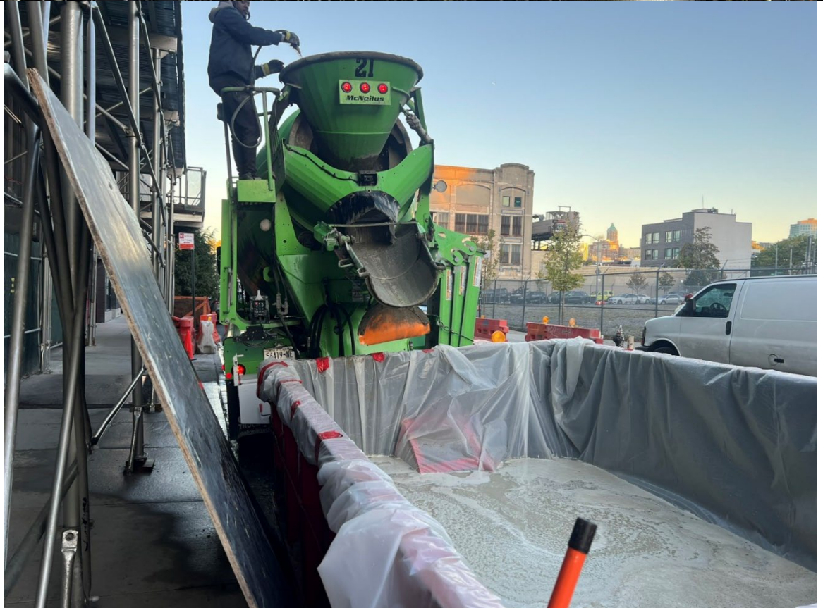
Photo 2- Representative photo of a concrete washout box.
