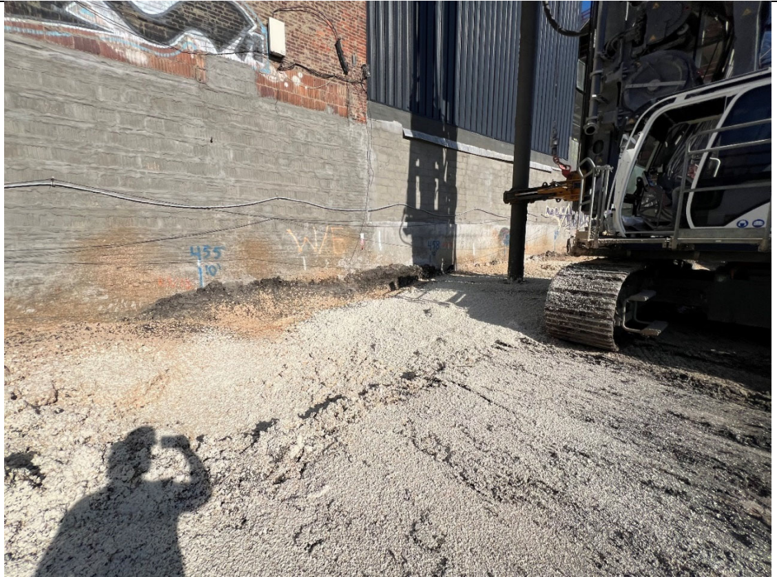
Photo 1- Representative photo of ISS Drilling area covered with ATMOS foam.
