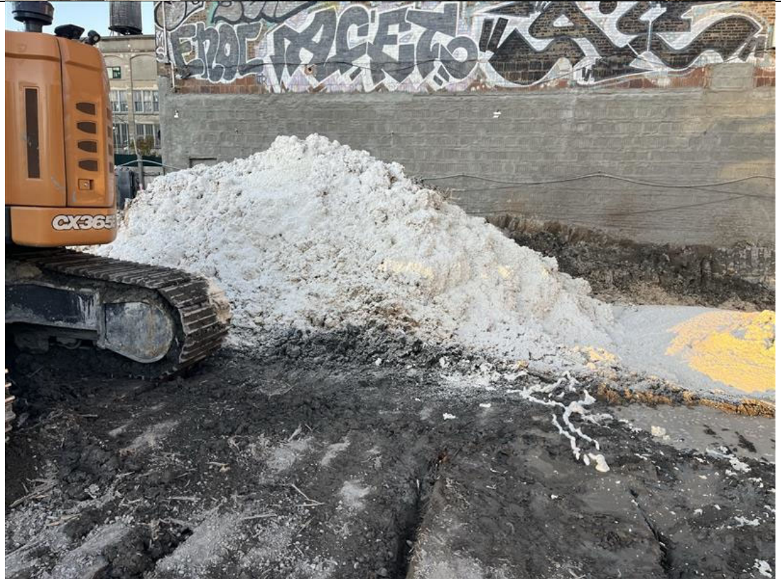
Photo 4- Representative photo of the swell stockpile covered with ATMOS foam at the end of the day.
