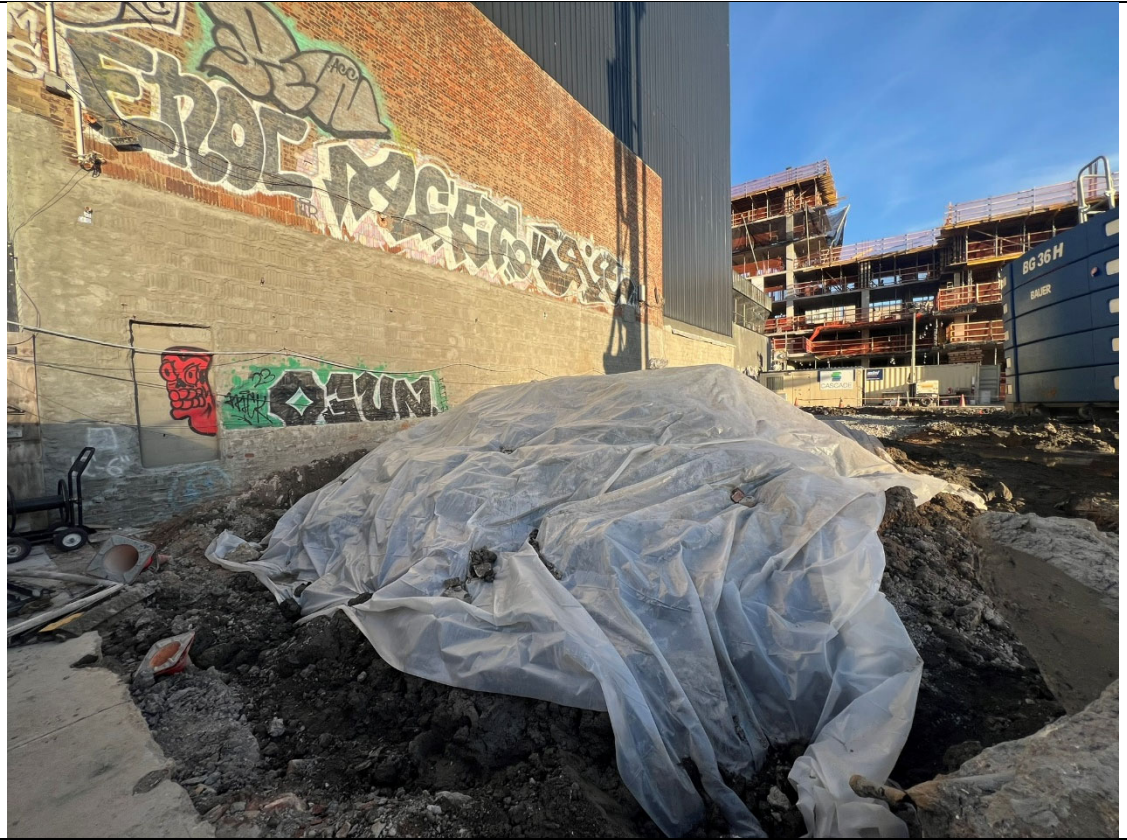
Photo 3- Representative Photo of covered soil stockpile at the end of the days activities.
