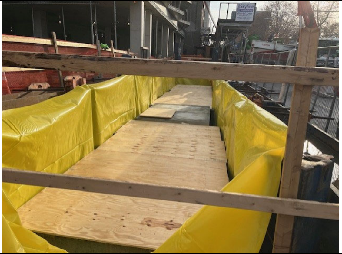
Photo 5- Representative photo of delivered ConEd Vault.
