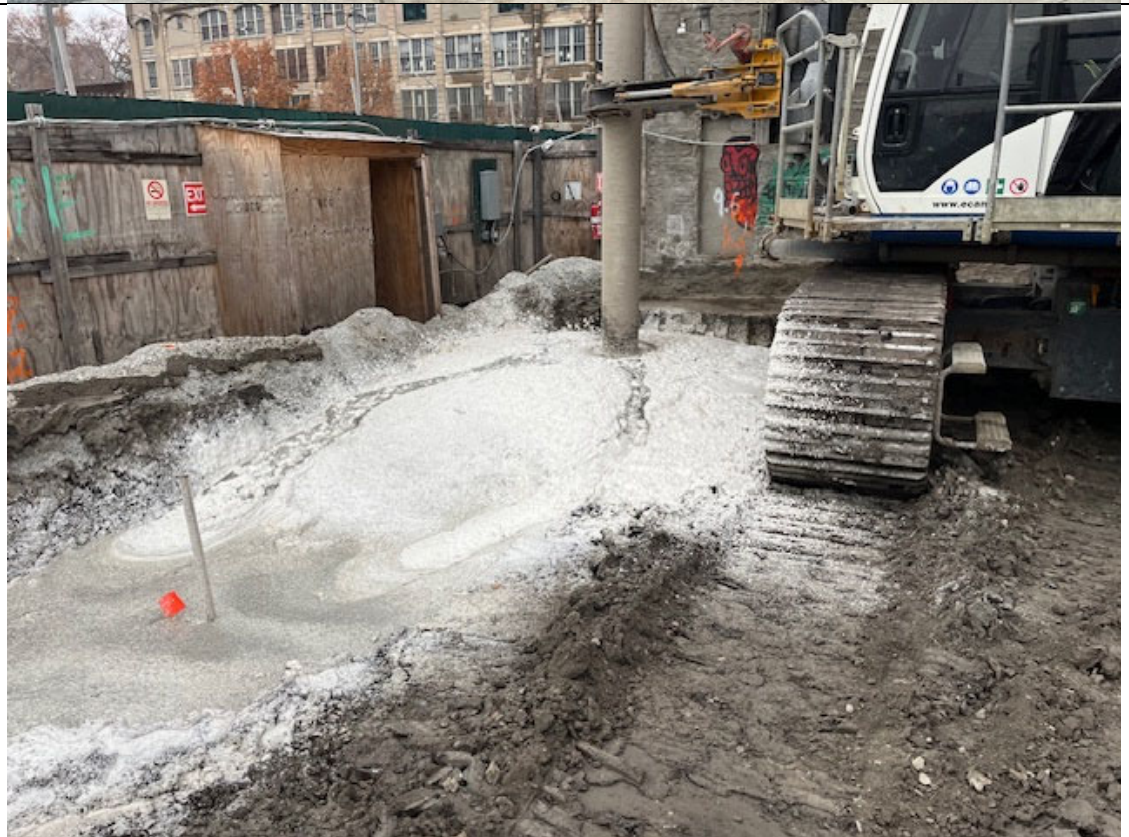
Photo 2- Representative photo of ISS installation.
