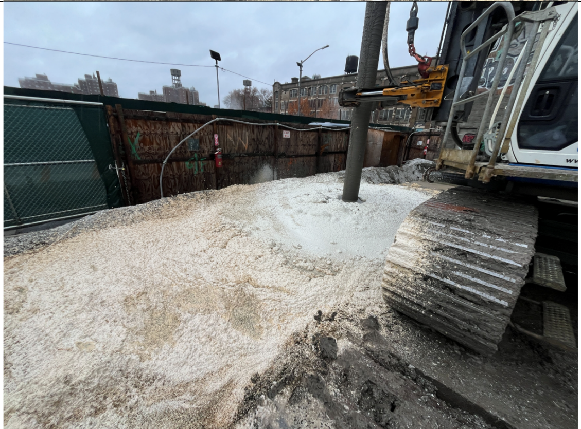
Photo 2- Representative photo of ISS installation.
