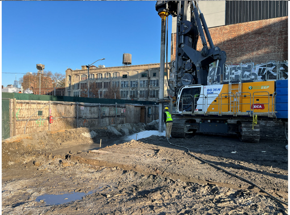
Photo 2- Representative photo of ISS installation.
