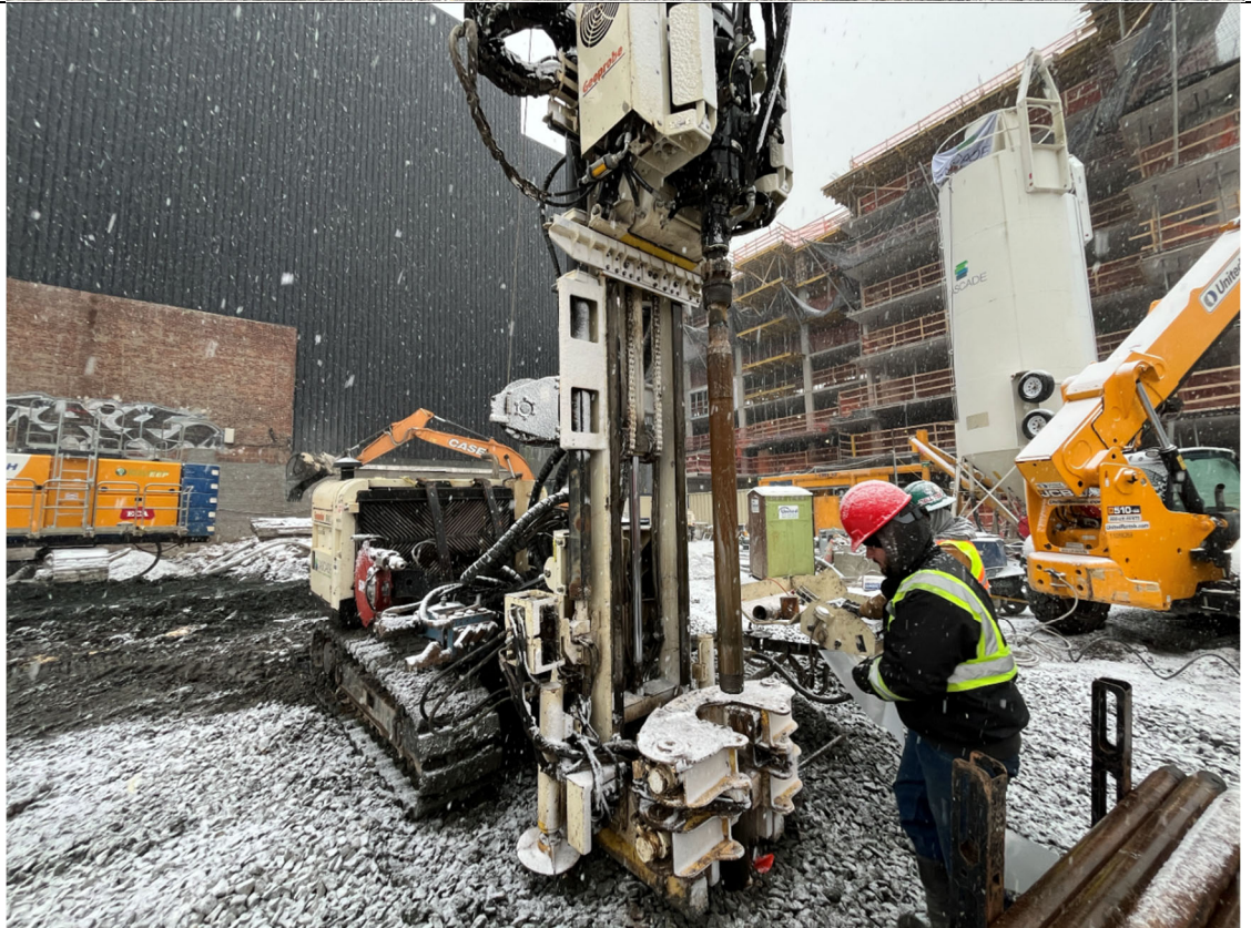
Photo 2- Representative photo of ADT coring 56-73 OL.
