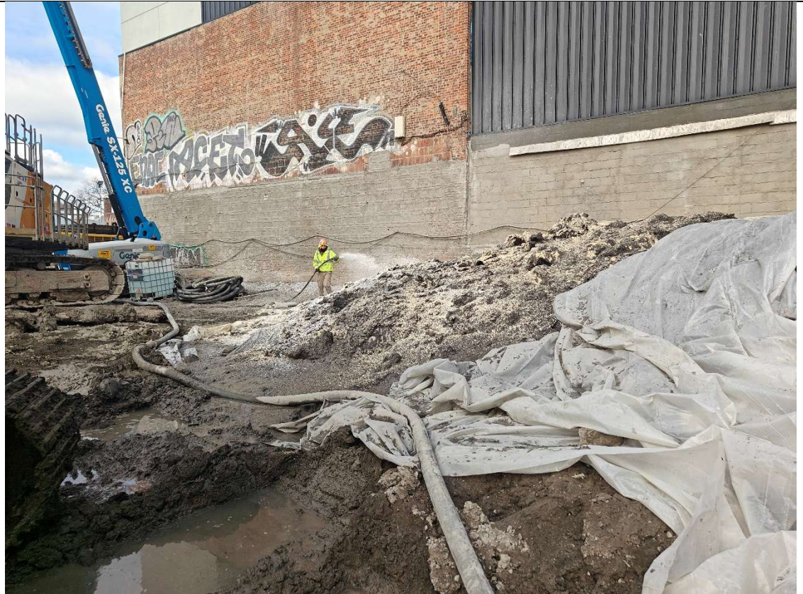
Photo 3- Representative photo of spraying swell stockpile.
