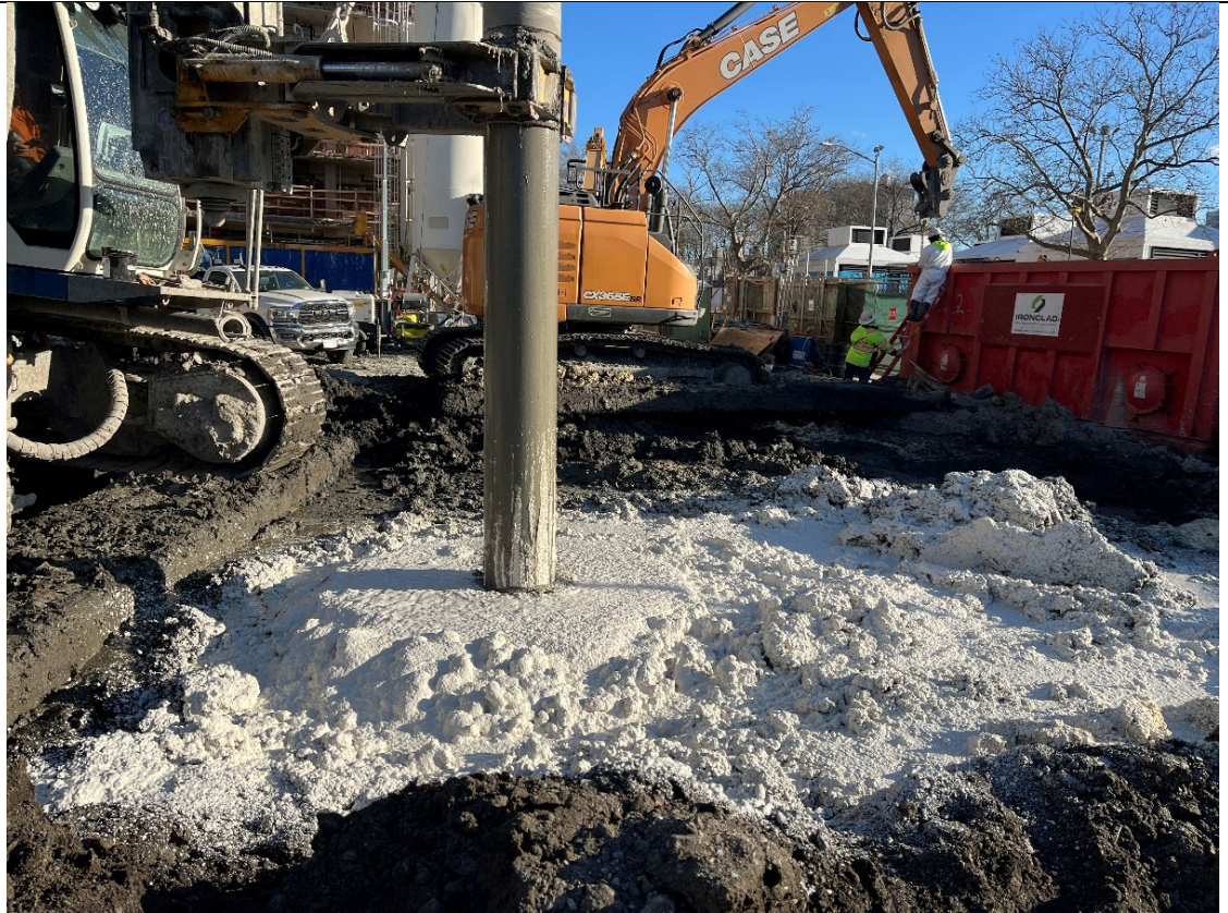
Photo 1- Representative photo of ISS installation.
