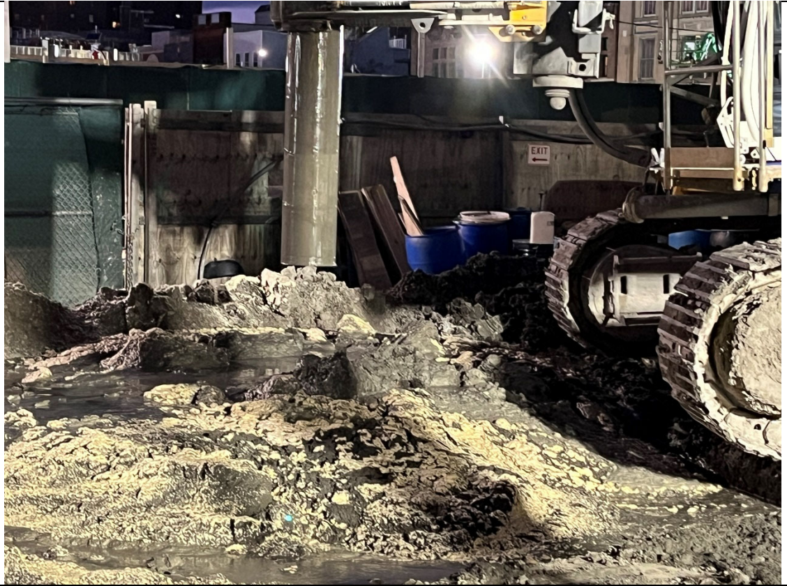
Photo 5- Representative photo of rig/ drill string failure.
