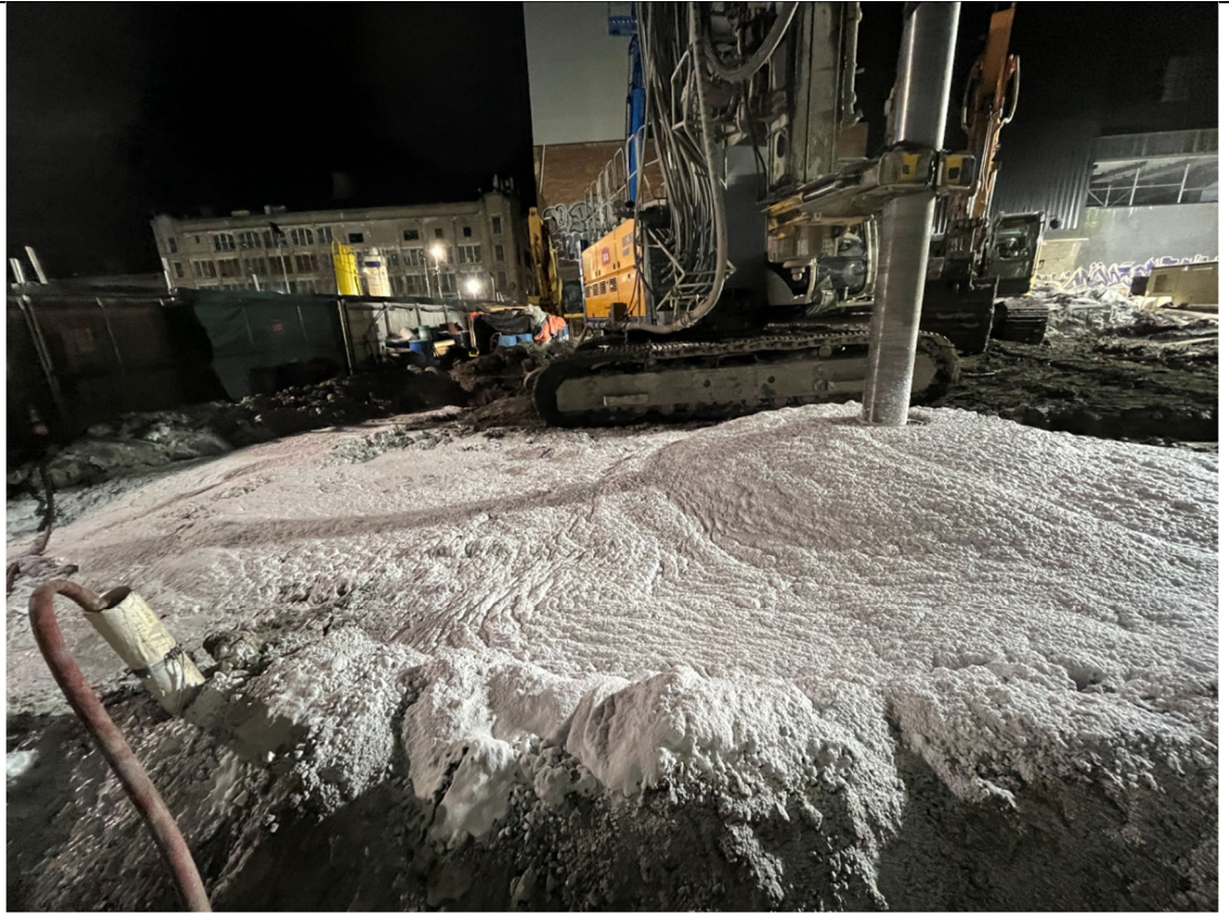
Photo 1- Representative photo of ISS installation.
