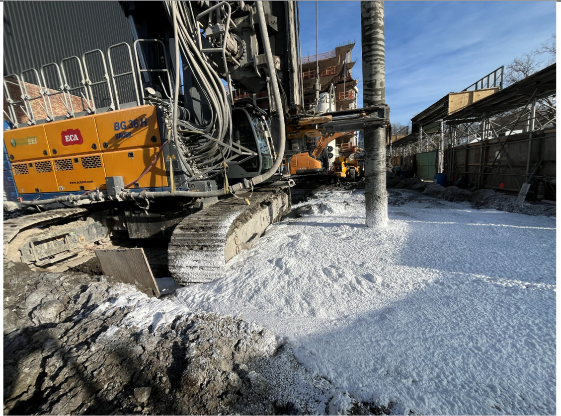
Photo 1- Representative photo of ISS installation.
