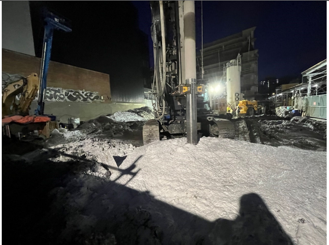
Photo 1- Representative photo of ISS installation.
