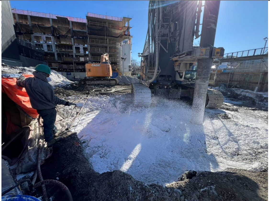
Photo 1- Representative photo of ISS installation.
