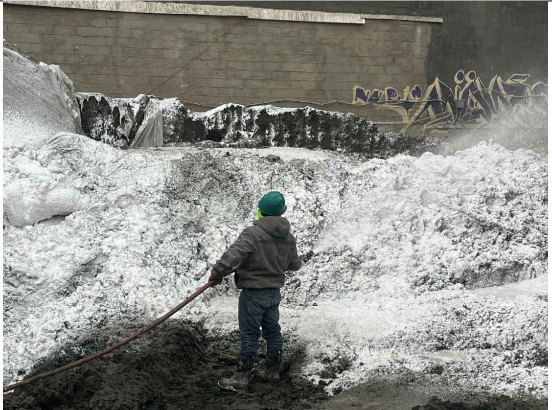
Photo 3- Representative photo of spraying the work area at the end of the day.
