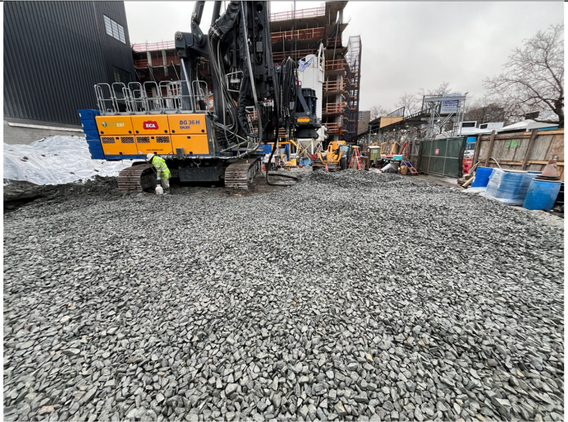
Photo 1- Representative photo of vehicle pad in the western portion of the site.
