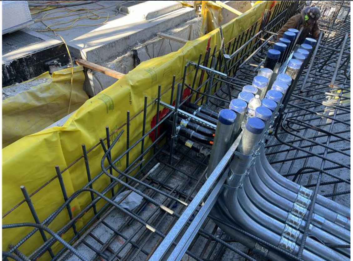
Photo 2- Representative photo of utility conduits sealed within the vapor barrier.
