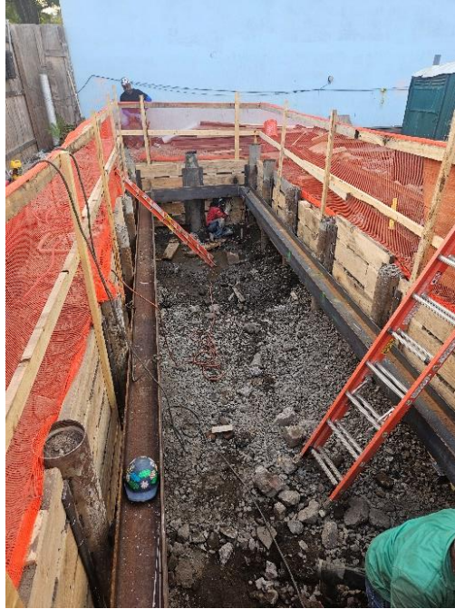
Photo 1: View of contractor welding I beams in the northeastern area of the Site, facing East.
