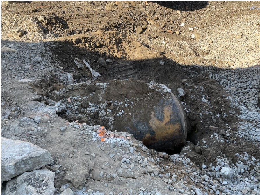
Photo 2: View of encountered UST in eastern portion of the site, facing West.
