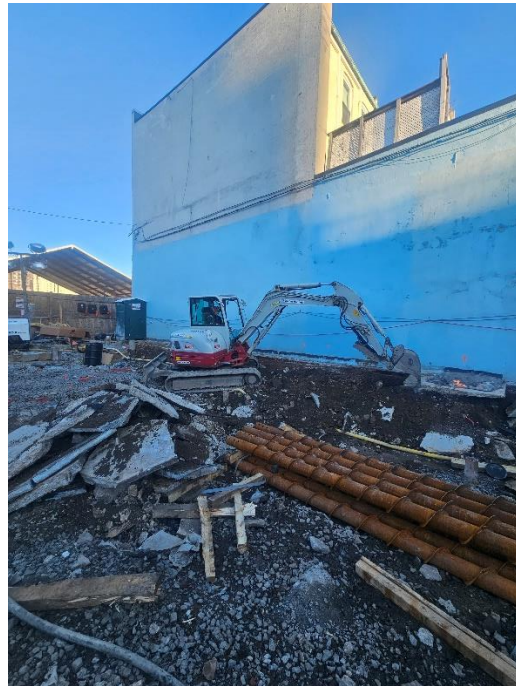
Photo 2: View of Blanco removing concrete slab in the eastern portion of the site, facing Northeast.
