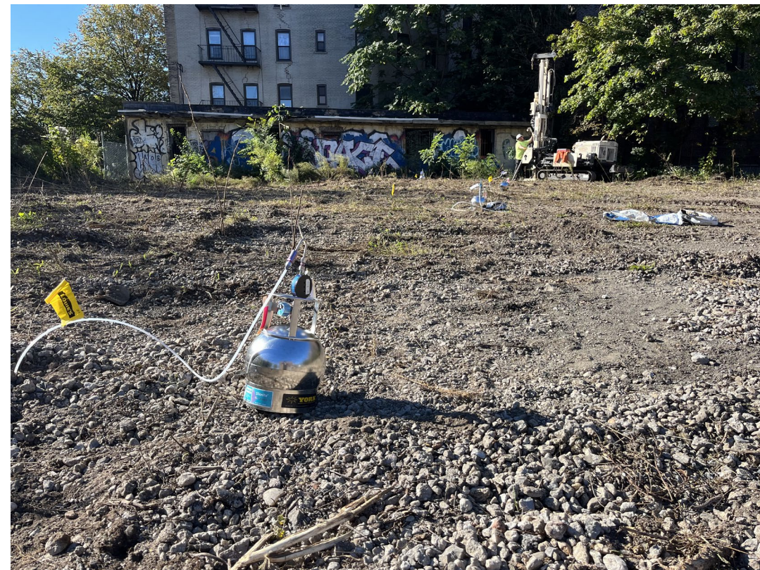
Summa canister connected to the soil vapor sampling implant
