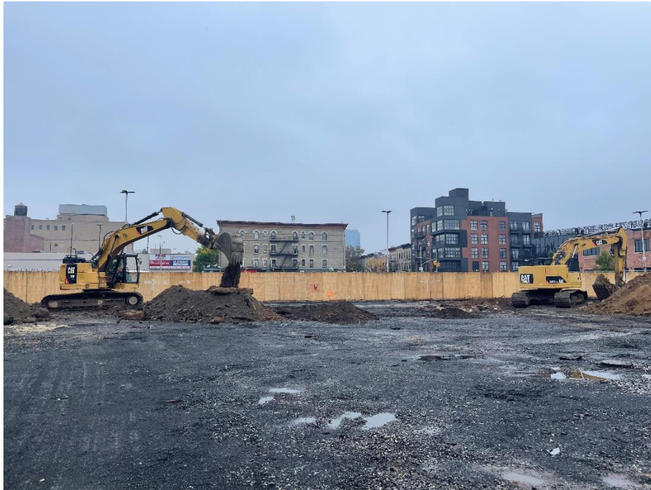
Photo 1: View of excavation for SOE installation along the perimeter of Lot 14, facing north.
