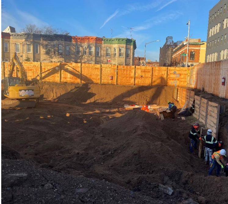
Photo 1: View of contractor installing lagging along the perimeter of Lot 14, facing west-southwest.
