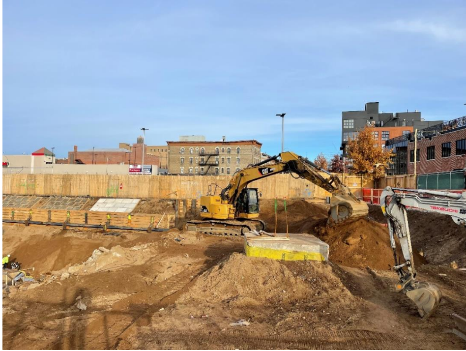
Photo 1: View of contractor grading Site soil along the perimeter of Lot 14, facing north.
