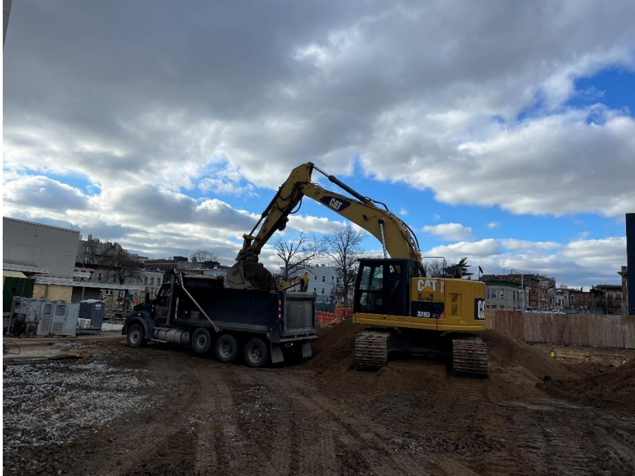
Photo 1: View of contractor loading soil for off-site disposal on Lot 14, facing southwest.
