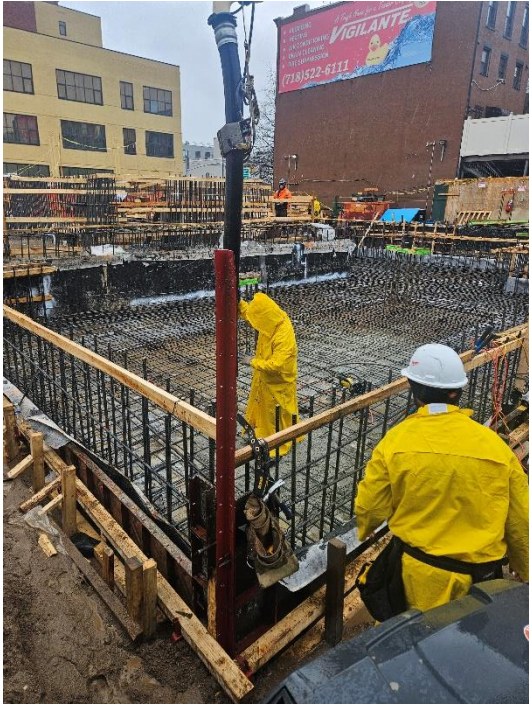
Photo 2: View of contractor pouring concrete for foundation elements in the western region of the Site.
