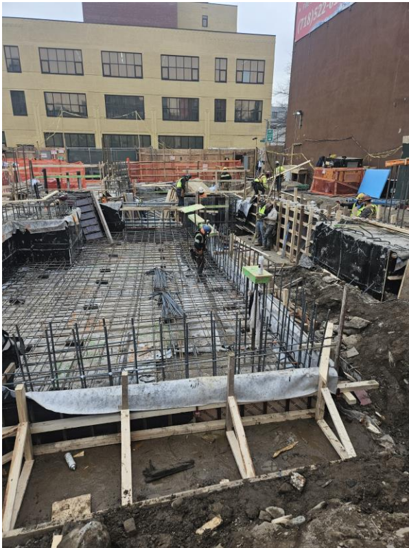
Photo 1: View of Site conditions in the eastern region of the Site, facing south.
