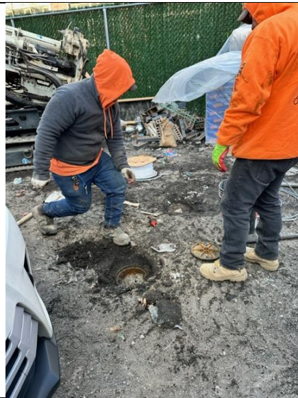
Interior Monitoring Well Location
