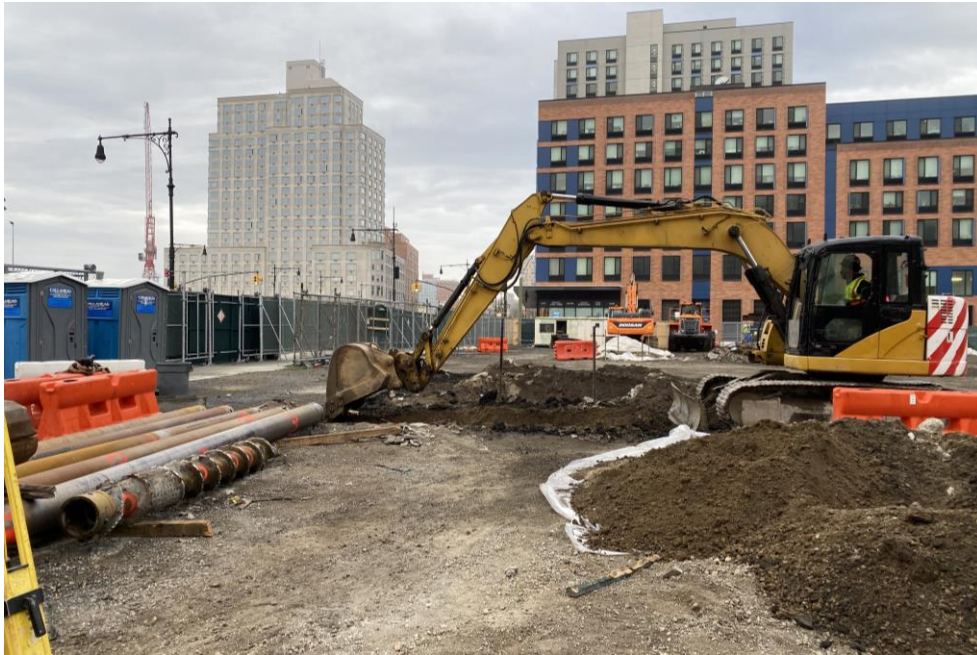
Photo 1: View of RYC Turbos Corp. excavating non-hazardous soil/fill in the southeastern part of the site (facing west).
