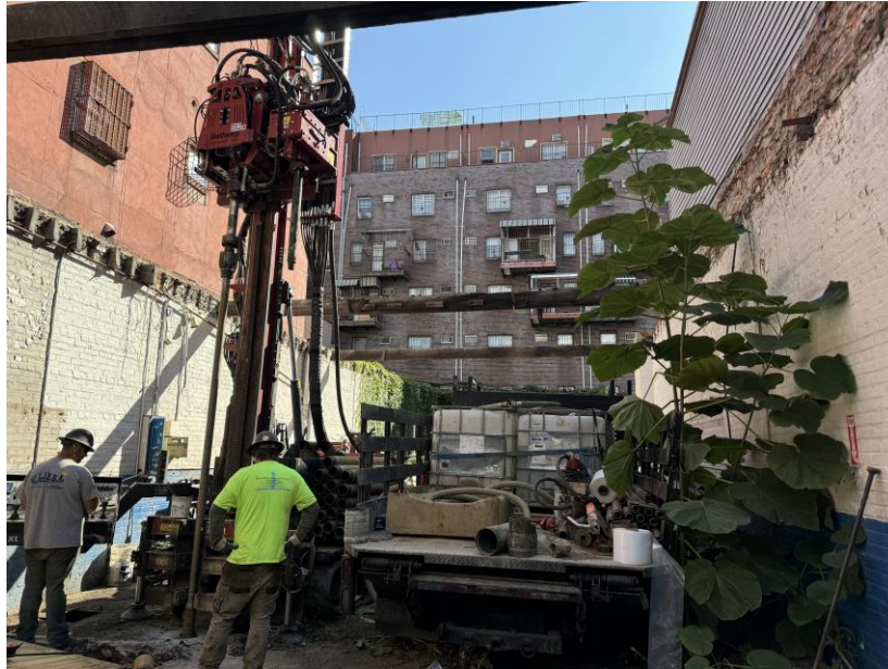
Photo 1: View of contractor installing soil boring SB-06 using a sonic drill rig, facing east.
