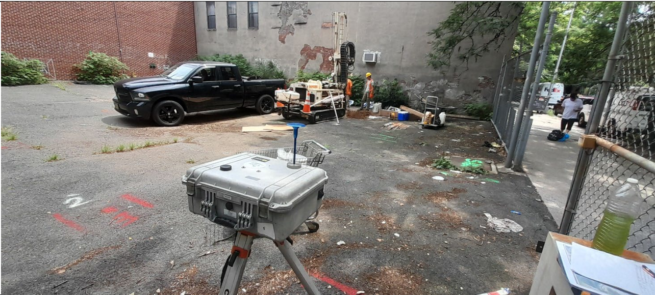
Photo 1: View from upwind CAMP station – Trinity installing RXSB-4.
