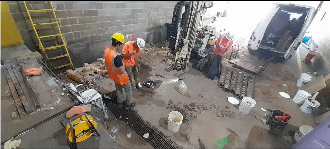
Photo 4: View of flush mount well set at RXMW-5.
