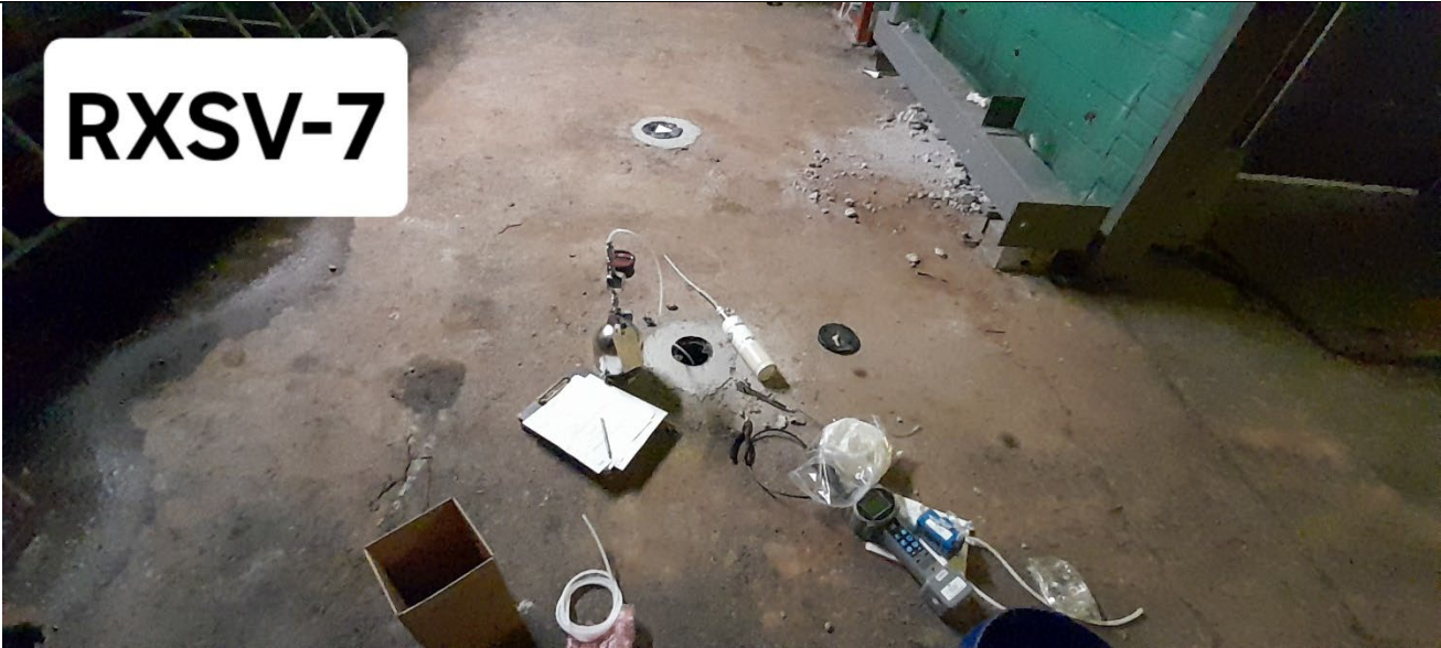
Photo 3: Soil vapor collection at RXSV-7.
