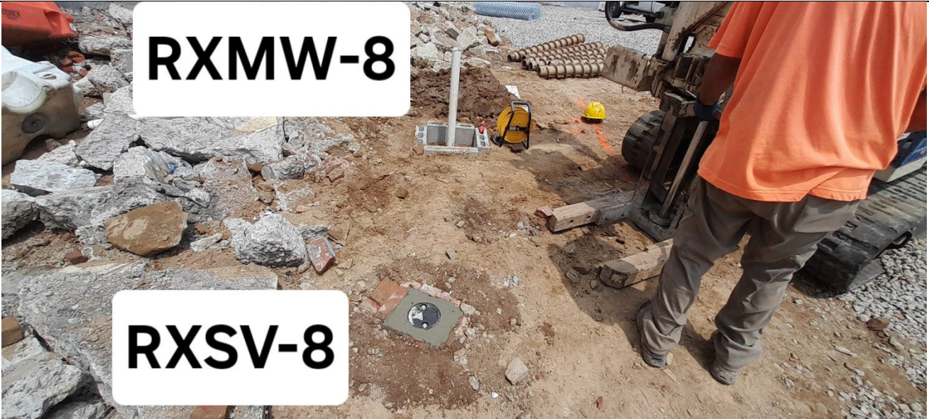
Photo 3: View of Trinity compleing RXMW-8 with flush mount well box adjacent to RXSV-8.
