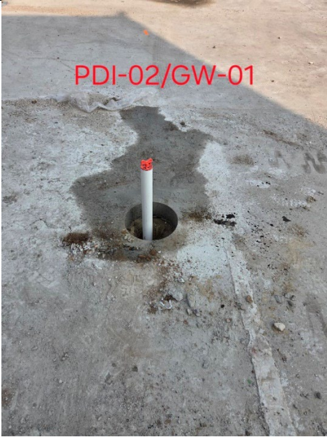
Photo 1: PDI-02 Installed on site and developed.
