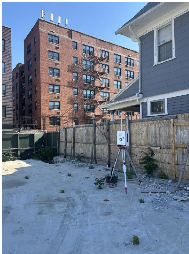
Photo 4: View of AQS1/Receptor 1 CAMP station, facing northeast.
