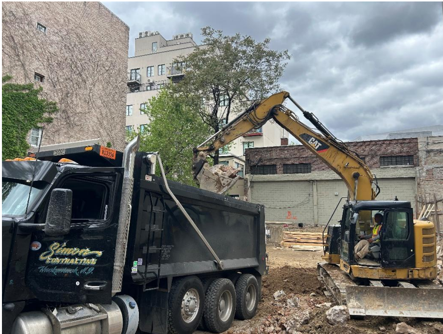
Photo 2: View of contractors loading a tri-axel truck with C&D materials, facing northwest.
