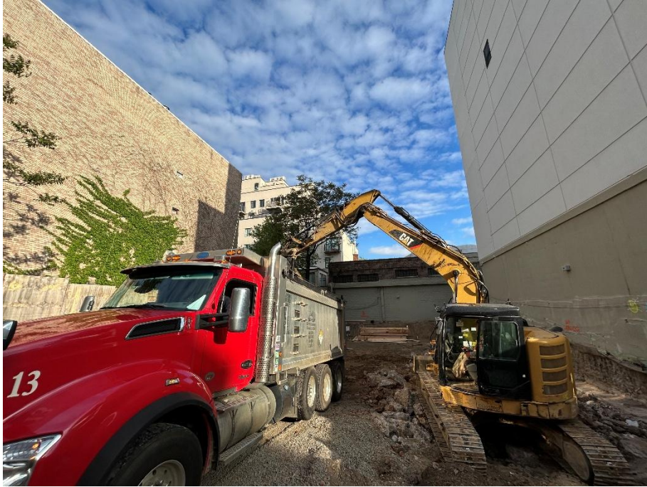
Photo 1: View of contractors loading a tri-axel truck with hazardous lead impacted soil, facing north.
