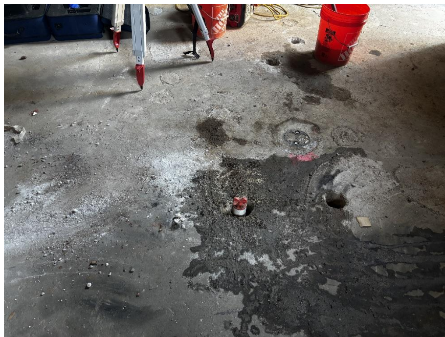
Photo 2: View of monitoring well MW01 in the northwestern part of the site (facing down).
