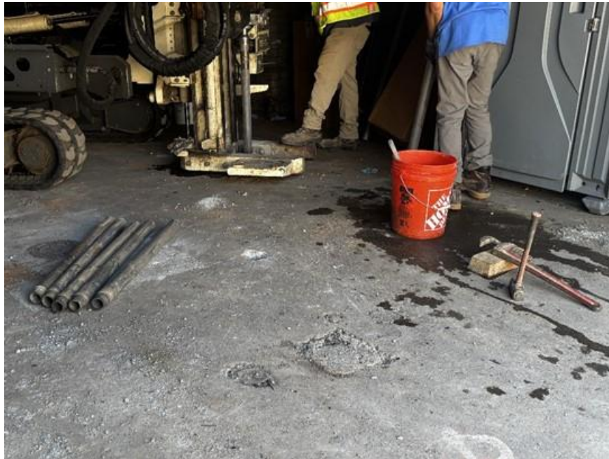
Photo 2: View of Ephase 2 advancing the soil boring location for monitoring well MW05 in the northeastern part of the site (facing southwest).
