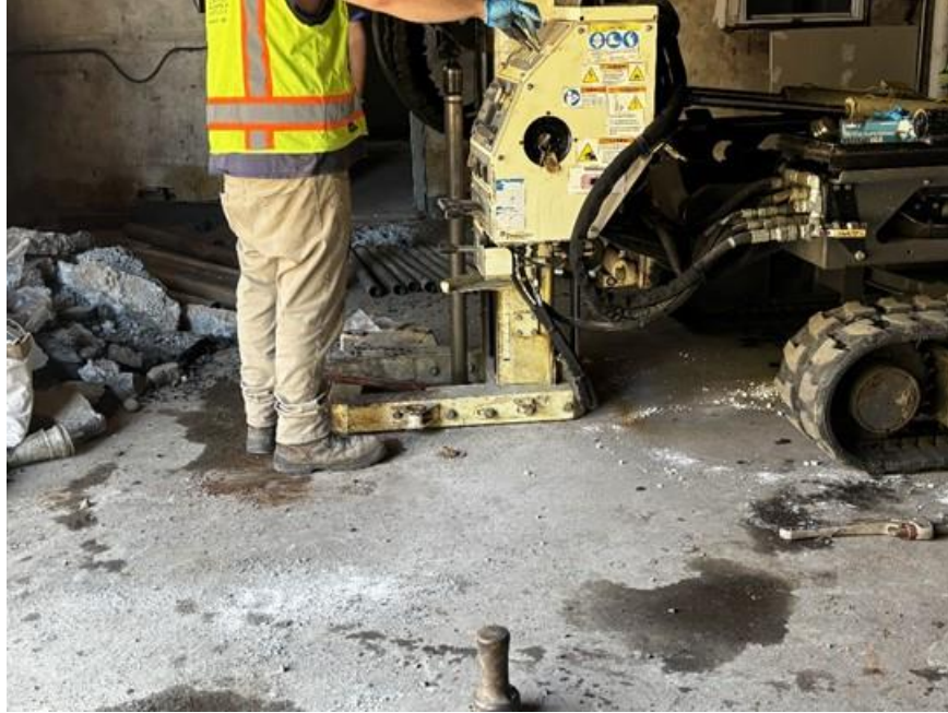
Photo 1: View of Ephase 2 advancing the soil boring location for monitoring well MW06 in the northeastern part of the site (facing east).
