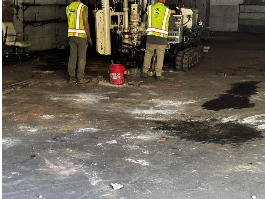
Photo 1: View of EPhase 2 advancing soil boring/monitoring well MW02 in the central part of the site (facing southeast).
