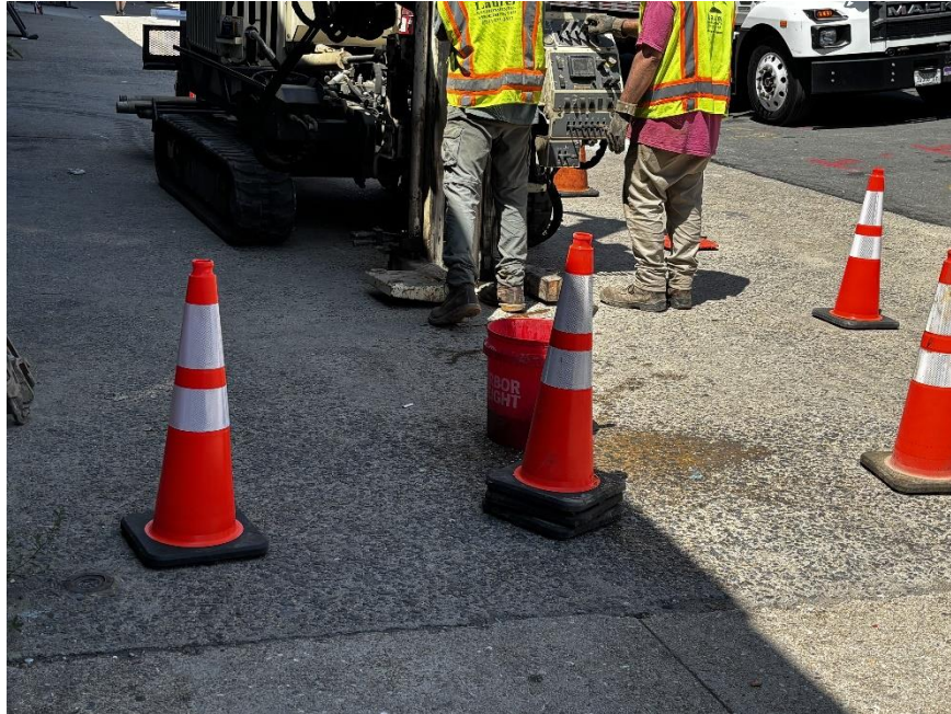
Photo 1: View of EPhase 2 advancing soil boring/monitoring well MW07 on the Montrose Avenue sidewalk (facing west).
