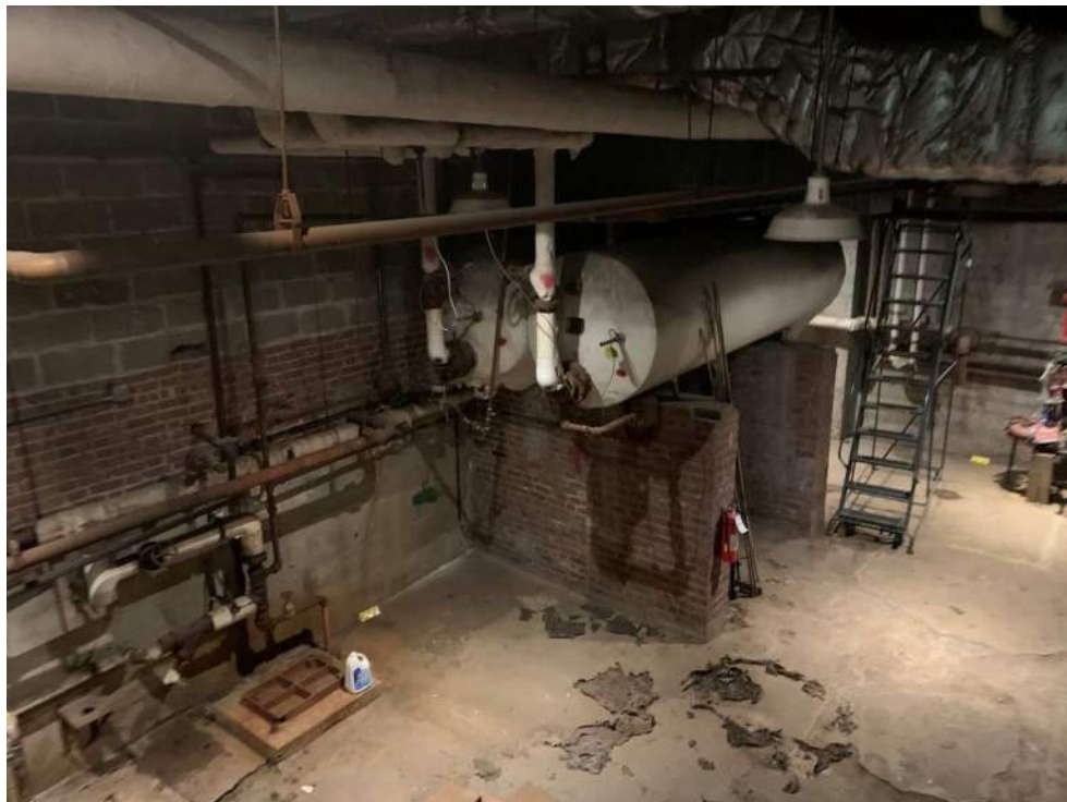
Photograph 35: View of boiler room in cellar of the Leviton building (facing southwest).
