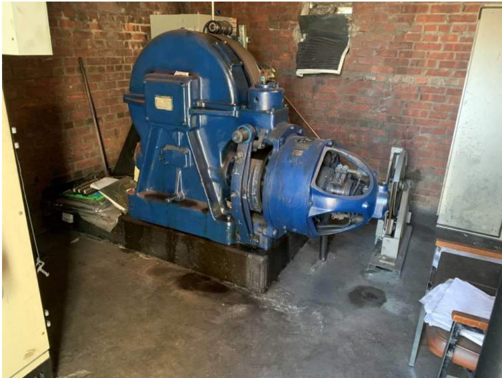
Photograph 16: View of elevator motor atop concrete slab in motor room on Blumberg roof (facing northwest).
