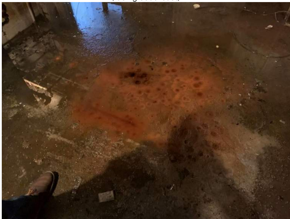
Photograph 24: View of rust-stained concrete and standing water in boiler room of Masin cellar (facing northwest).
