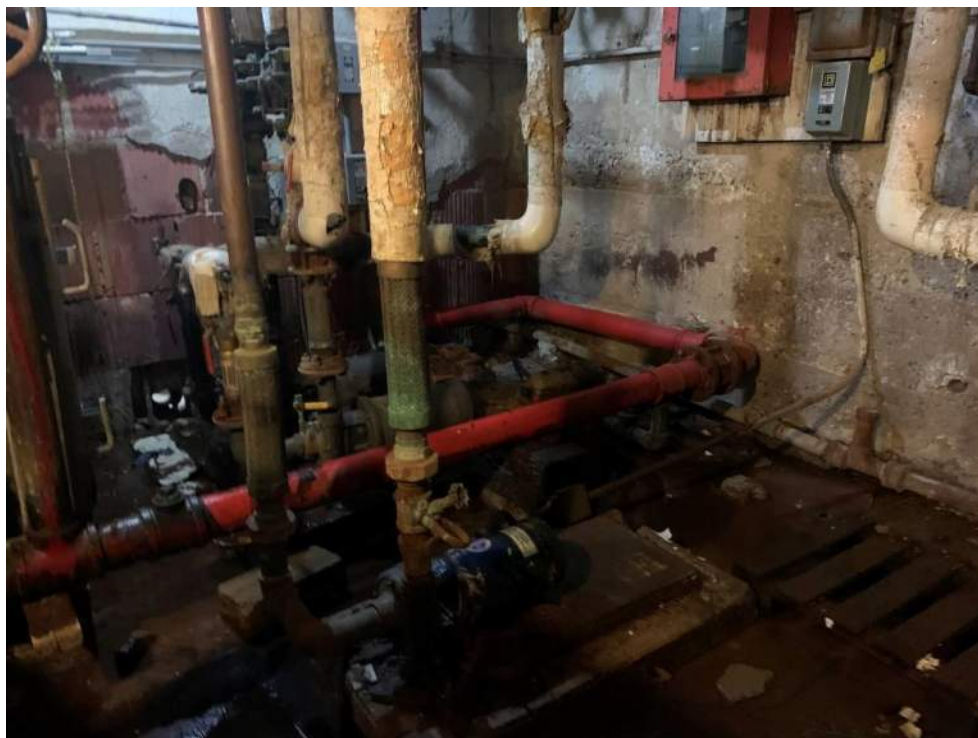
Photograph 11: View of leaking boiler in maintenance area of Blumberg building cellar (facing northeast).
