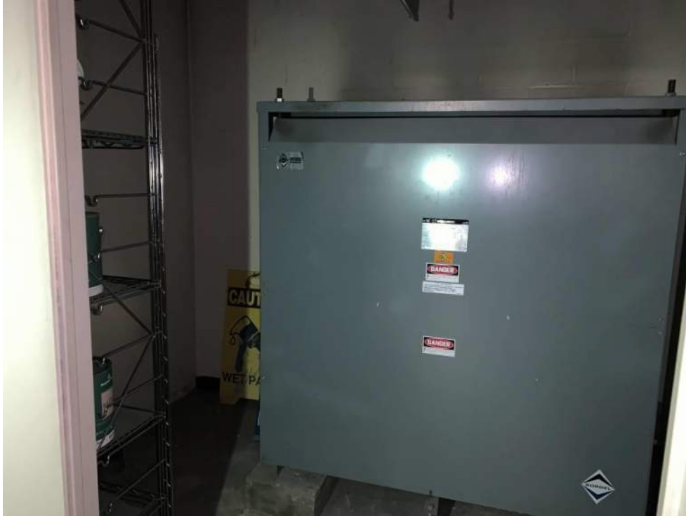
Photograph 21: View of a dry type transformer in cellar of the Masin building (facing east).
