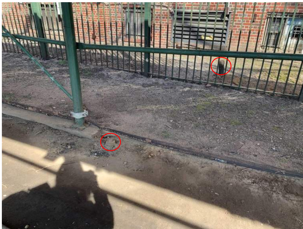
Photograph 47: View of fill port and vent pipe along Leviton exterior from Schenectady Avenue (facing northeast).
