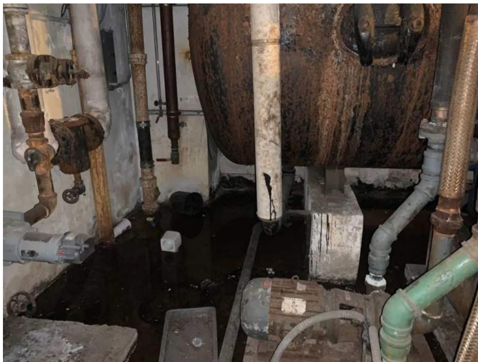
Photograph 25: View of hot water tank and standing water in boiler room of Masin cellar (facing east).
