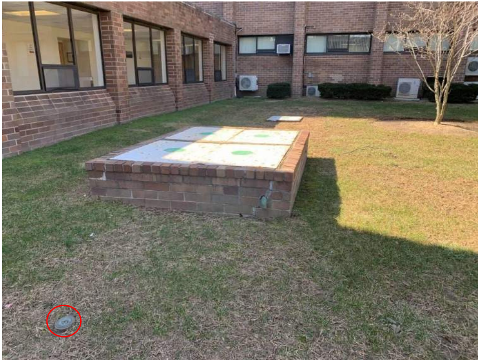
Photograph 41: View of 40,000 gallon No. 6 Fuel Oil underground storage tank (UST) vault and fill port on southern adjoining property in courtyard (facing west).
