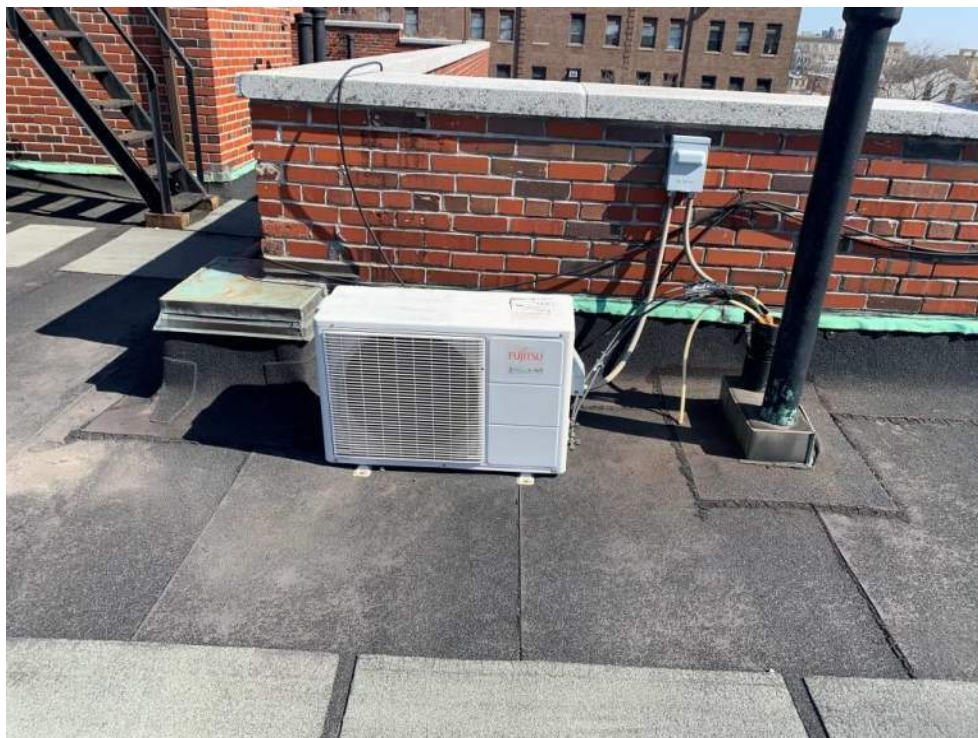
Photograph 37: View of DC Inverter air conditioning unit on the roof of the Leviton building (facing south).
