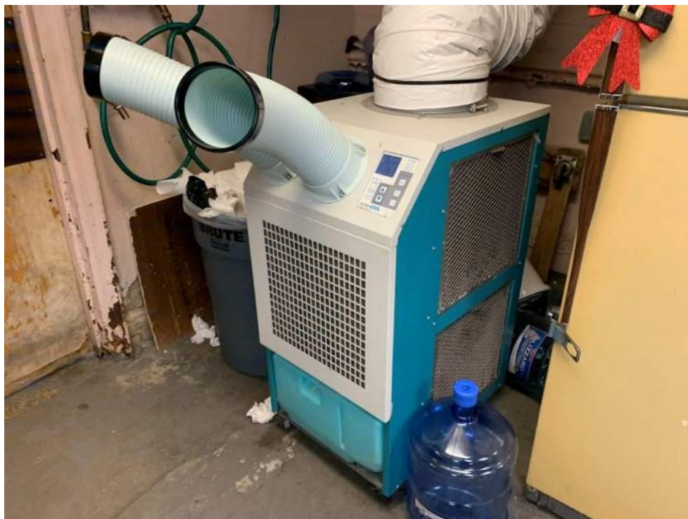
Photograph 3: View of portable air conditioning unit in partial cellar of the LeFrak building (facing east).
