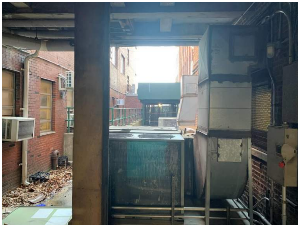
Photograph 17: View of a heating, ventilation and air conditioning (HVAC) unit between Masin and Blumberg buildings (facing east).
