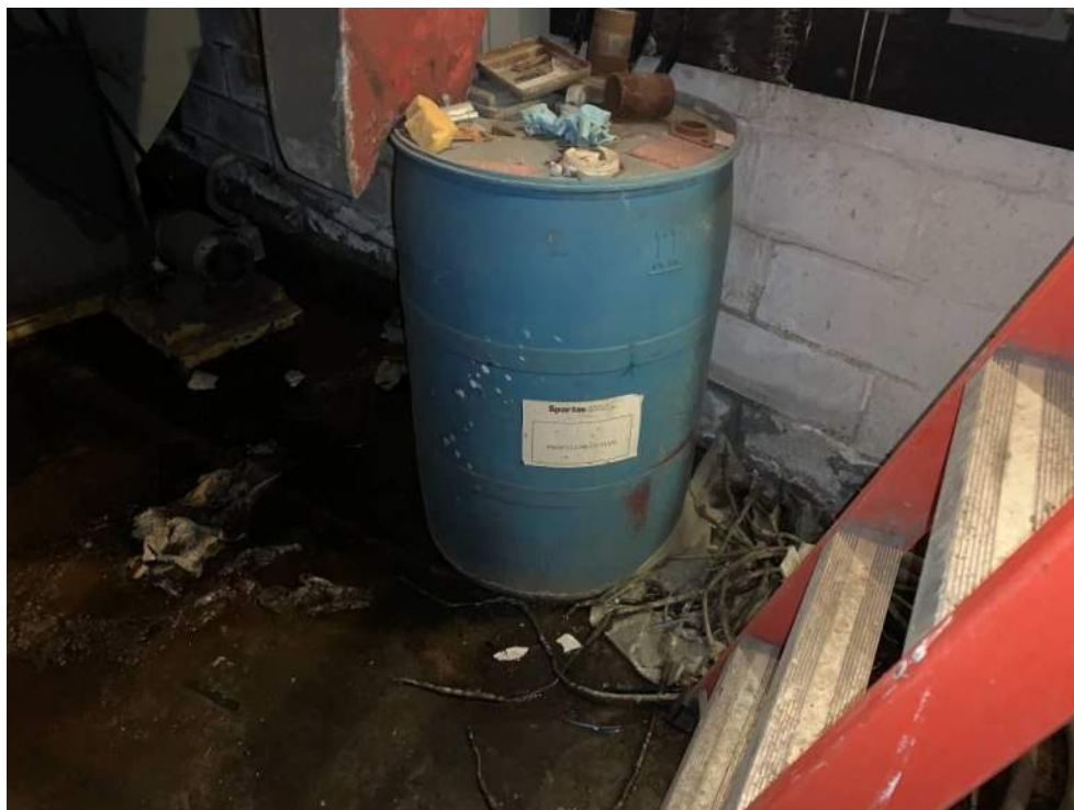
Photograph 23: View of plastic 55-gallon drum of propylene glycol in boiler room of Masin cellar (facing southeast).
