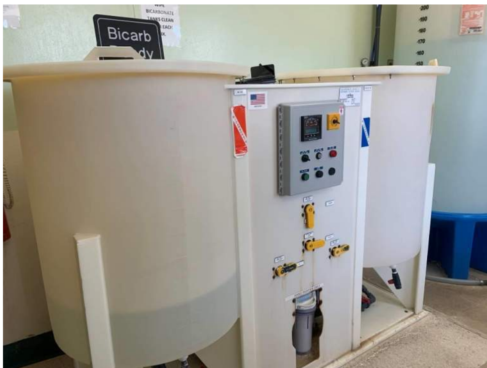
Photograph 12: View of bicarbonate tanks in dialysis water treatment room on the fifth floor of the Blumberg building (facing northeast).
