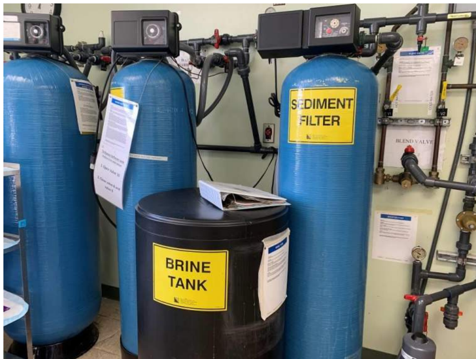
Photograph 13: View of sediment filter, carbon tanks, and brine tank in dialysis room on the fifth floor of the Blumberg building (facing west).
