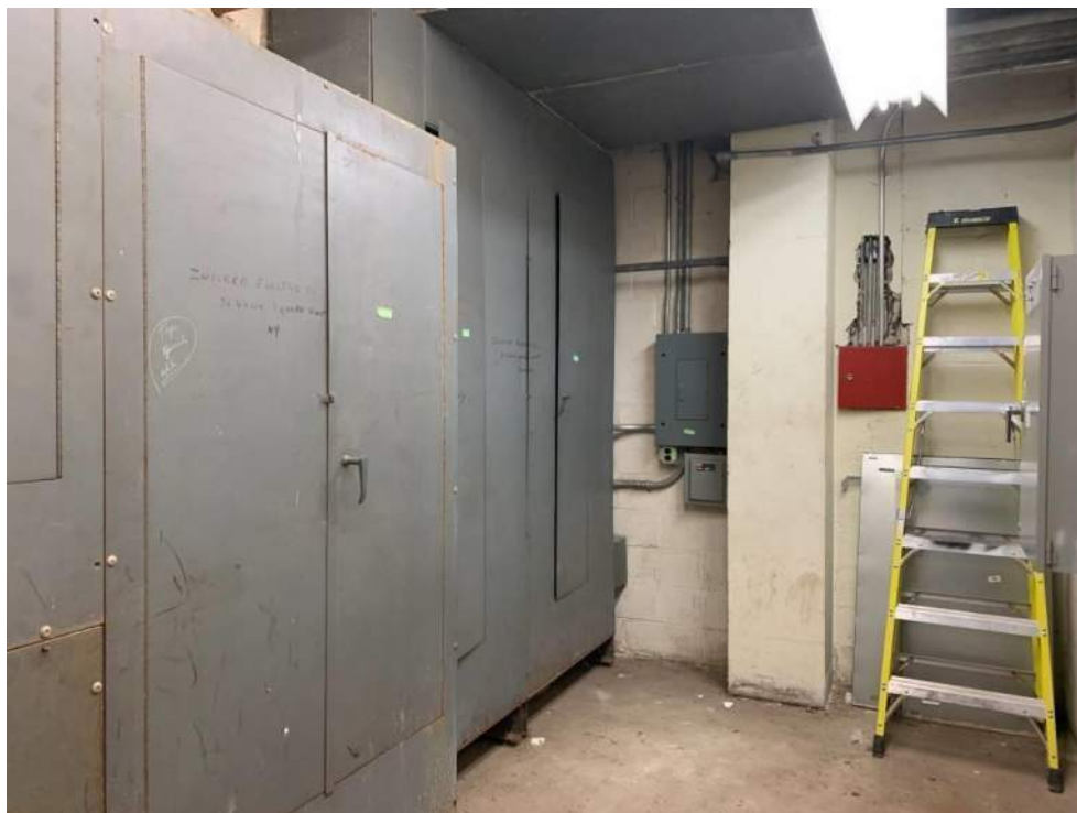
Photograph 19: View of electrical power boxes in cellar of the Masin building (facing north).
