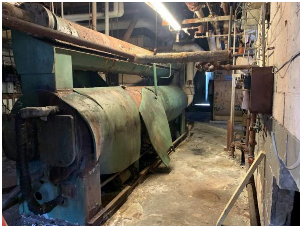
Photograph 31: View of hot water tank in maintenance area on roof of the Masin building (facing east).
