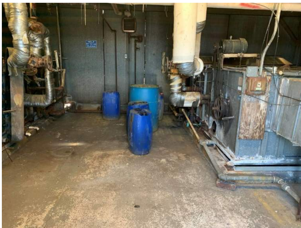
Photograph 32: View of plastic drums with unknown contents and HVAC system in maintenance area on roof of the Masin building (facing south).
