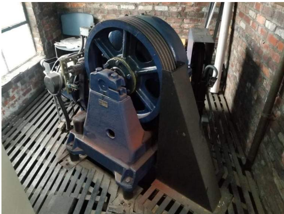
Photograph 6: View of elevator motor located on the roof of the Leviton building (facing south).
