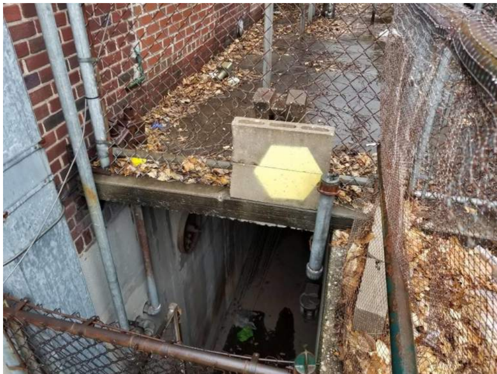
Photograph 31: View of a diesel tank fill port on the southeastern adjoining building (facing north).
