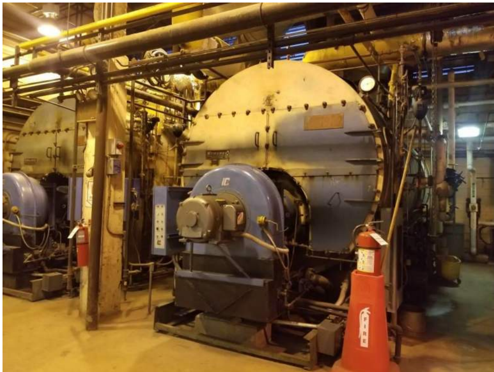
Photograph 30: View of two of three natural gas powered boilers that provide steam to the Kingsbrook Jewish Medical Center campus, located on the ground floor of the southeastern adjoining building (facing southwest).
