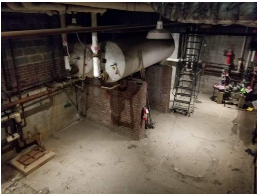
Photograph 8: View of boiler room in cellar of the Leviton building (facing southwest).
