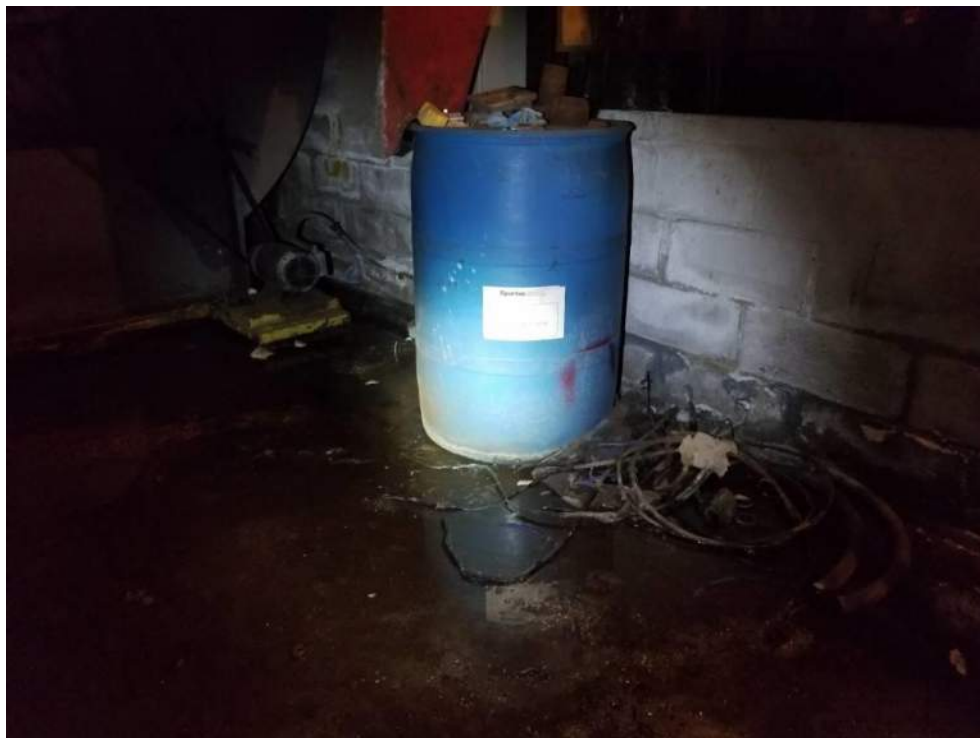
Photograph 19: View of plastic 55-gallon drum of propylene glycol in boiler room of Masin cellar (facing southeast).
