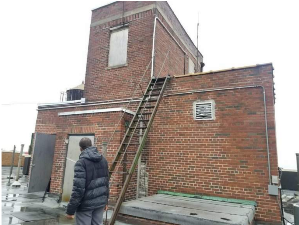
Photograph 25: View of elevator motor rooms on the roof of the Blumberg building (facing northeast).
