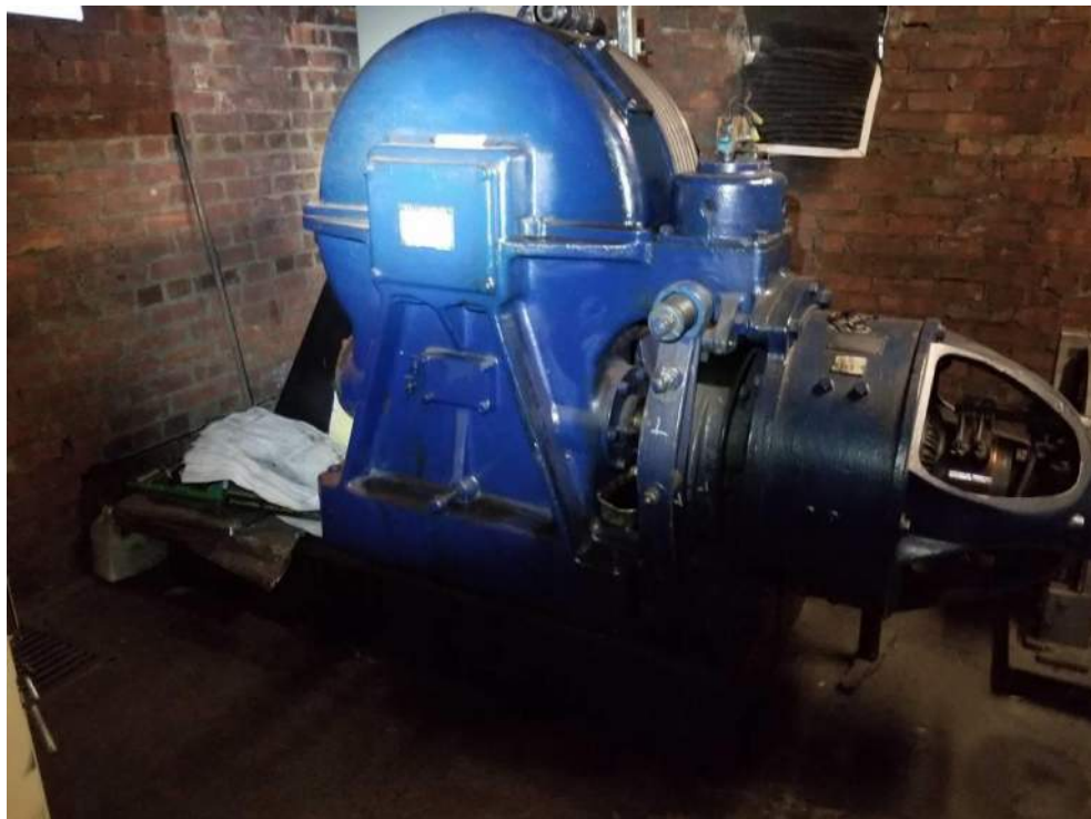
Photograph 26: View of elevator motor atop concrete slab in motor room on Blumberg building roof (facing northwest).
