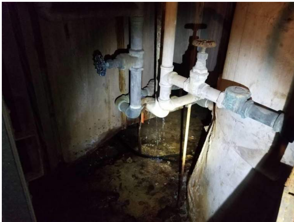
Photograph 21: View of leaking pipes in the former boiler room in the cellar of the Masin building (facing north).
