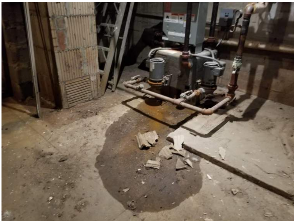
Photograph 7: View of water and rust staining beneath a pump in the cellar of the Leviton building (facing south).
