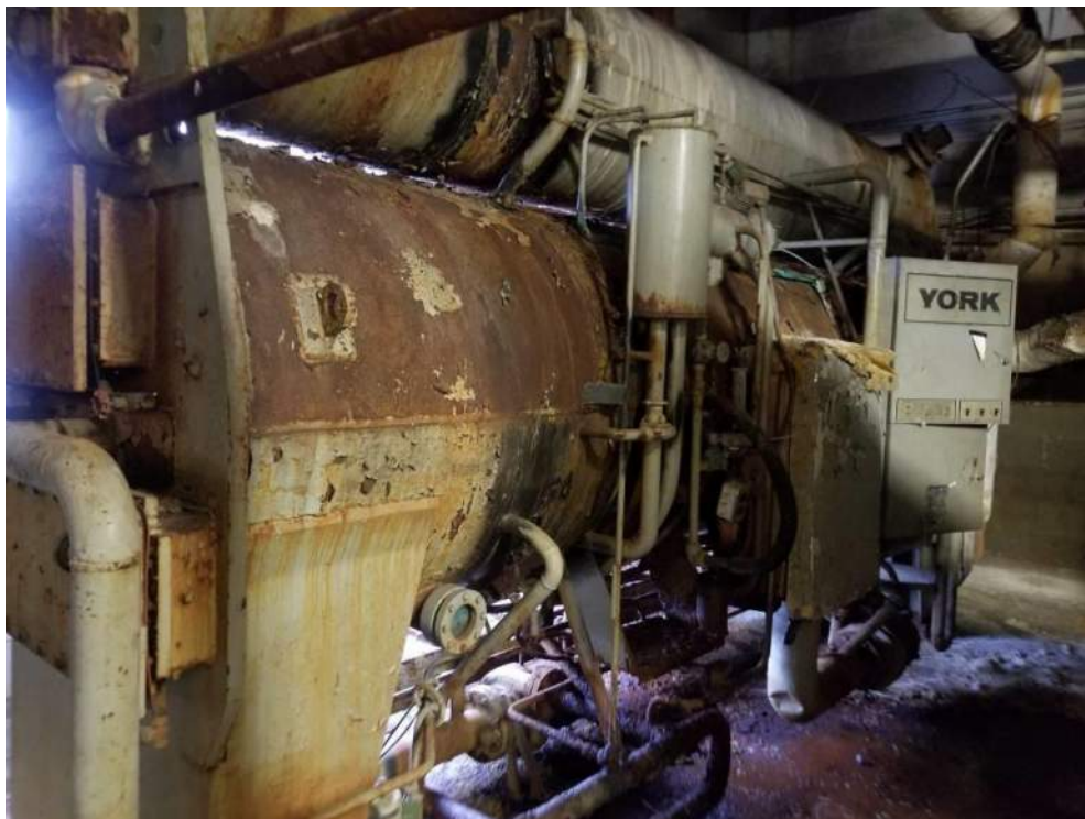
Photograph 10: View of inactive heating, ventilation, and air conditioning (HVAC) equipment on the roof of the Leviton building (facing northwest).
