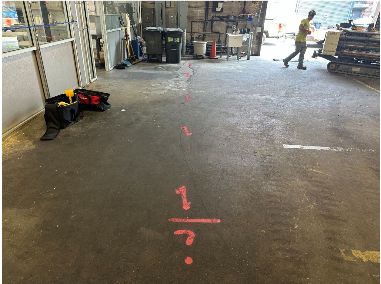
Photo 2 – Electric line detected but its signal dropped off midway through the building. It was marked out in red paint and labeled 'E'.
