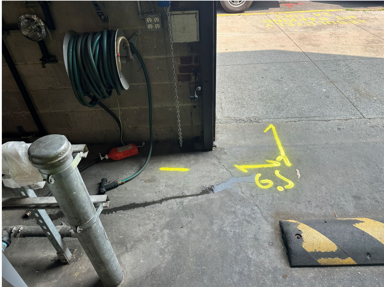
Photo 3 – Gas service line detected connecting from the road to the building. Once the gas line connected to the main it ran overhead.
