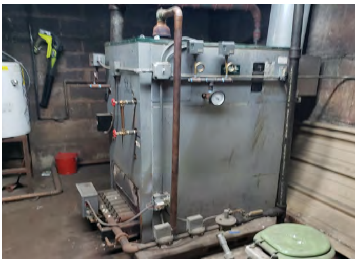
Natural gas-fired boiler in basement
