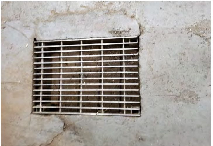
Drain in basement
