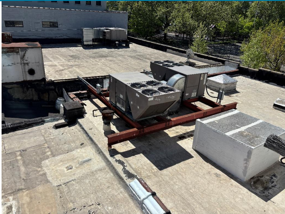
Photo 3: View of HVAC system on roof of Lot 48 of the site, facing southwest.
