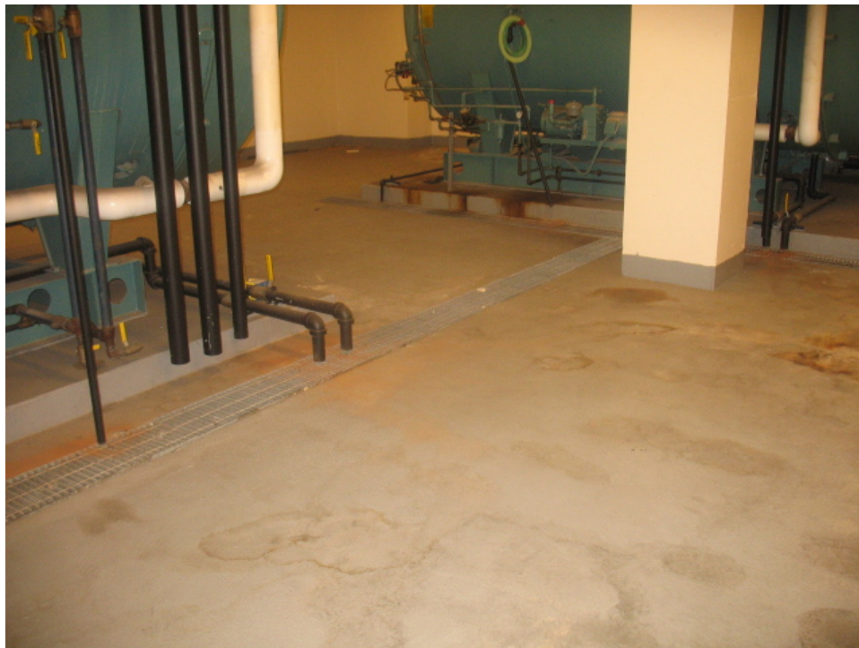
Photograph No. 4: View of surface cover inside the boiler room of River Place II.
