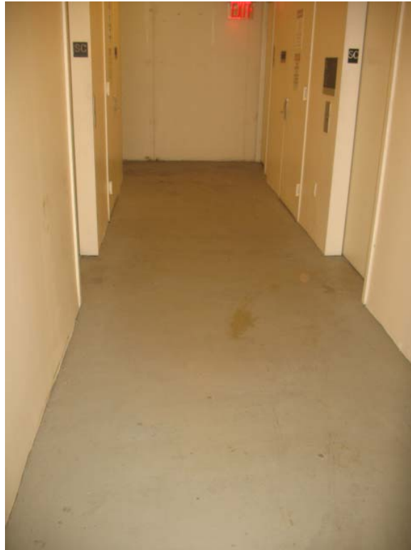
Photograph No. 3: View of hallway floor in lower level of River Place II.
