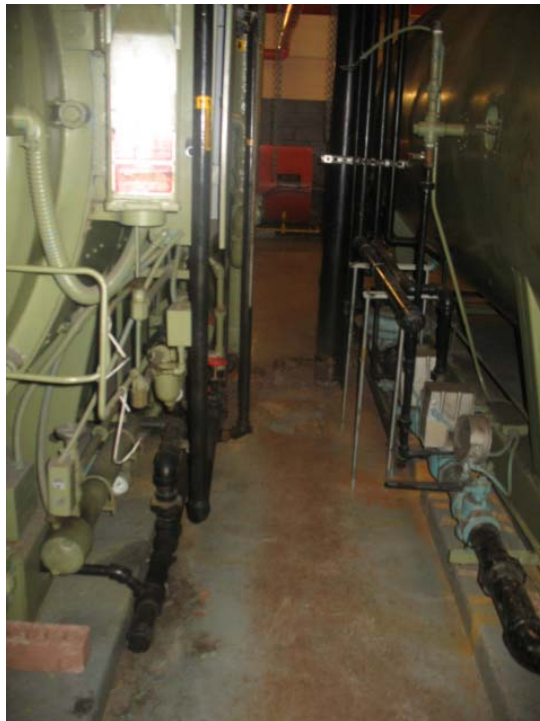
Photograph No. 16: View of concrete floor in mechanical room of River Place I.
